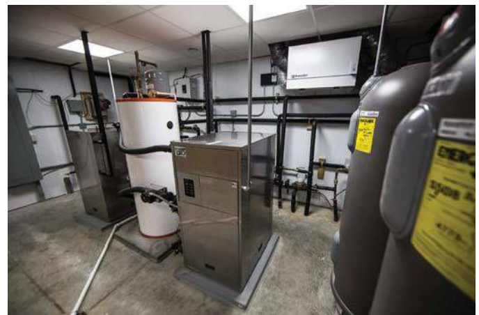
The mechanical room in the lower level houses the water heater, ERV and geothermal system that keeps the house at a comfortable, consistent temperature year-round.
