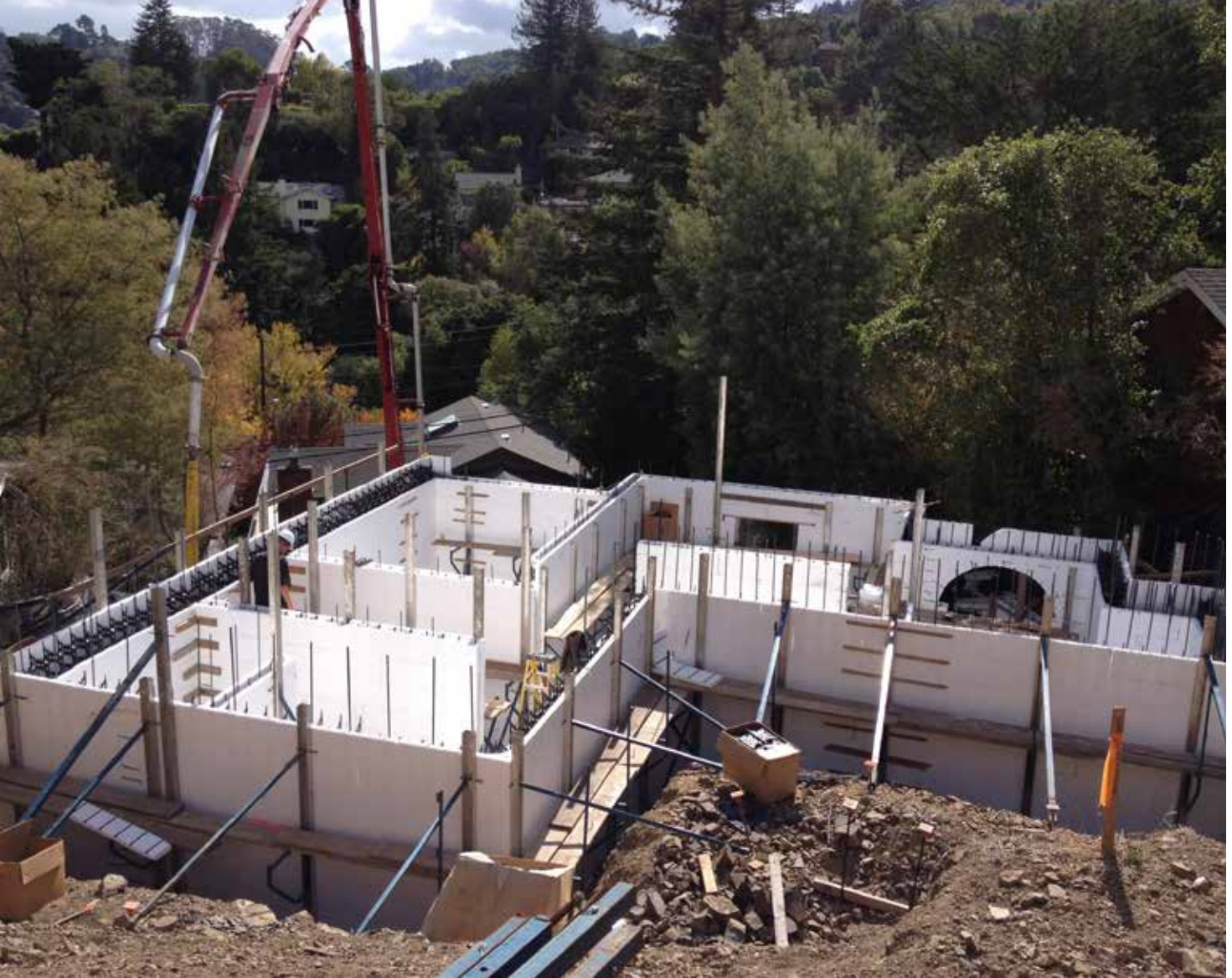
IntegraSpec Insulating Concrete Forms were used to construct both exterior and interior walls of the three-story custom home. ICF use: 25,000 square feet. Photo courtesy Nicholas Nikiforuk, IntegraSpec.
